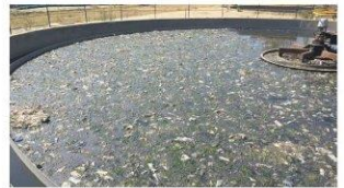
Clarifier not working
