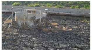
Clarifier not working
