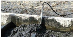
Chlorinator gets mixed and treated.
