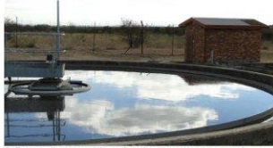
6 Days later the plant works normal. Sludge removed to drying beds.
