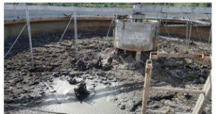
Clarifier not working
