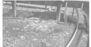
Clarifier not working
