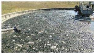
Clarifier not working
