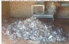
Pumpstation debris from pumpstation screens inside pumpstation.
