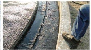
Clarifier not working
