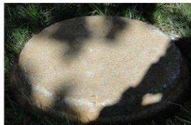
Standard manhole covers to be replaced with lockable covers
