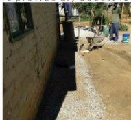
Yard drained and crusher stone laid to provide dry access to house
